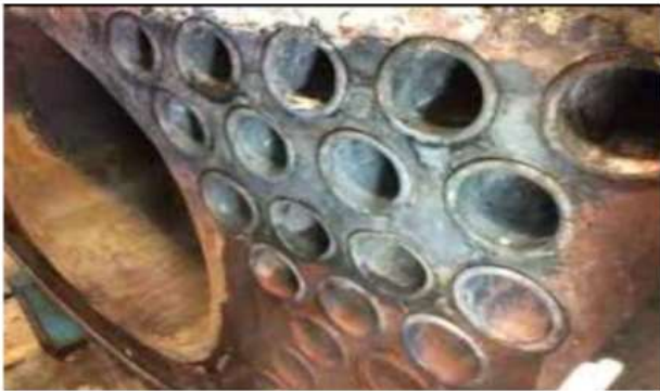
Fig. 4. Plugging of Bank Tubes of Boiler-II SGP NFL Naya Nangal.
