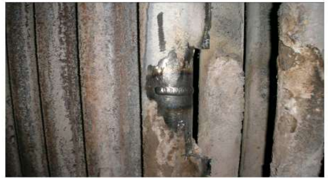
Fig. 2. Economizer Tubes of Boiler-I SGP NFL Naya Nangal.
